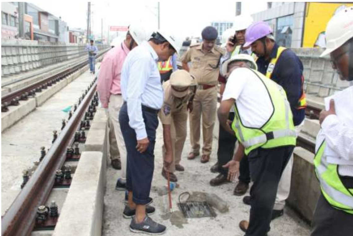
MD, HMRL Mr. NVS Reddy inspecting the rain water drainage arrangements on Metro Rail viaduct between Madhapur and Hitec city Metro stations with L&THRHL engineers on Saturday (26.08.2017)
