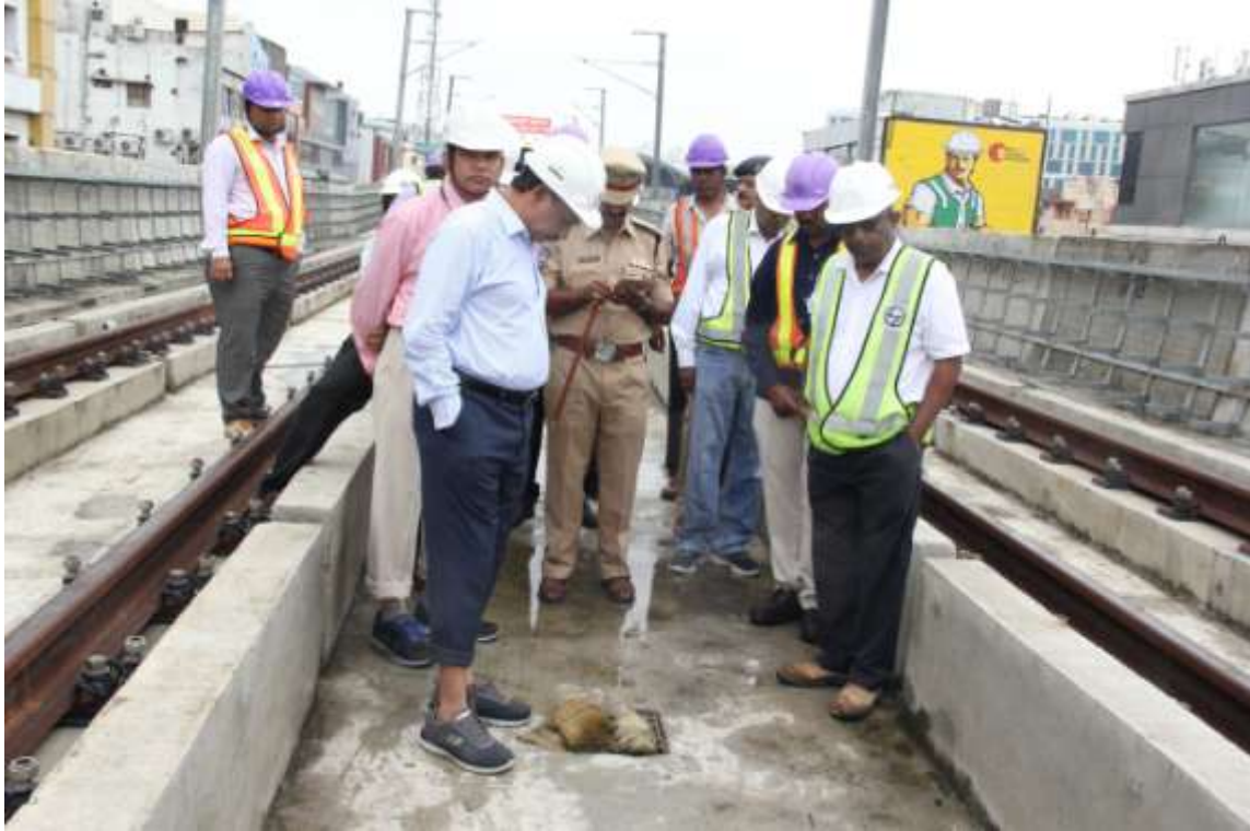
MD, HMRL Mr. NVS Reddy inspecting the rain water drainage arrangements on Metro Rail viaduct between Madhapur and Hitec city Metro stations with L&THRHL engineers on Saturday (26.08.2017)
