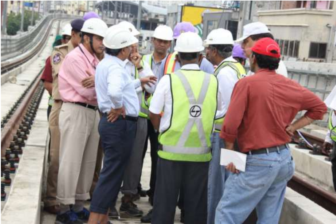
MD, HMRL Mr. NVS Reddy discussing the rain water drainage arrangements on Metro Rail viaduct between Madhapur and Hitec city Metro stations with L&THRHL engineers on Saturday (26.08.2017)
