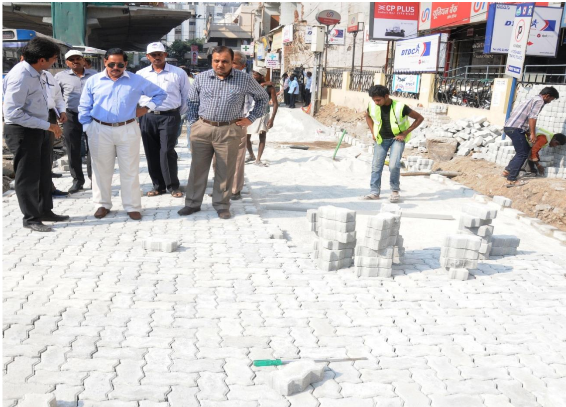
MD, HMRL Mr. NVS Reddy inspecting road restoration works with paver blocks at Khairatabad Metro station area on October 13, 2016 (Thursday). CE, HMRL Mr Md. Ziauddin is to his left.
