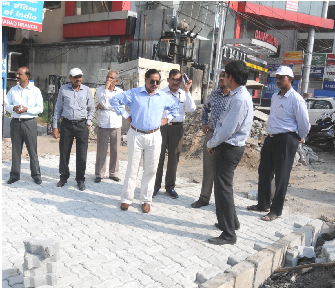
MD, HMRL Mr. NVS Reddy inspecting road restoration works with paver blocks at Khairatabad Metro station area on October 13, 2016 (Thursday)
