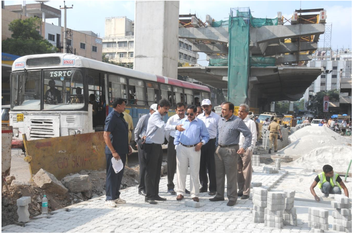
MD, HMRL Mr. NVS Reddy inspecting road restoration works with paver blocks at Khairatabad Metro station area on October 13, 2016 (Thursday). CE, HMRL Mr Md. Ziauddin is to his left.
