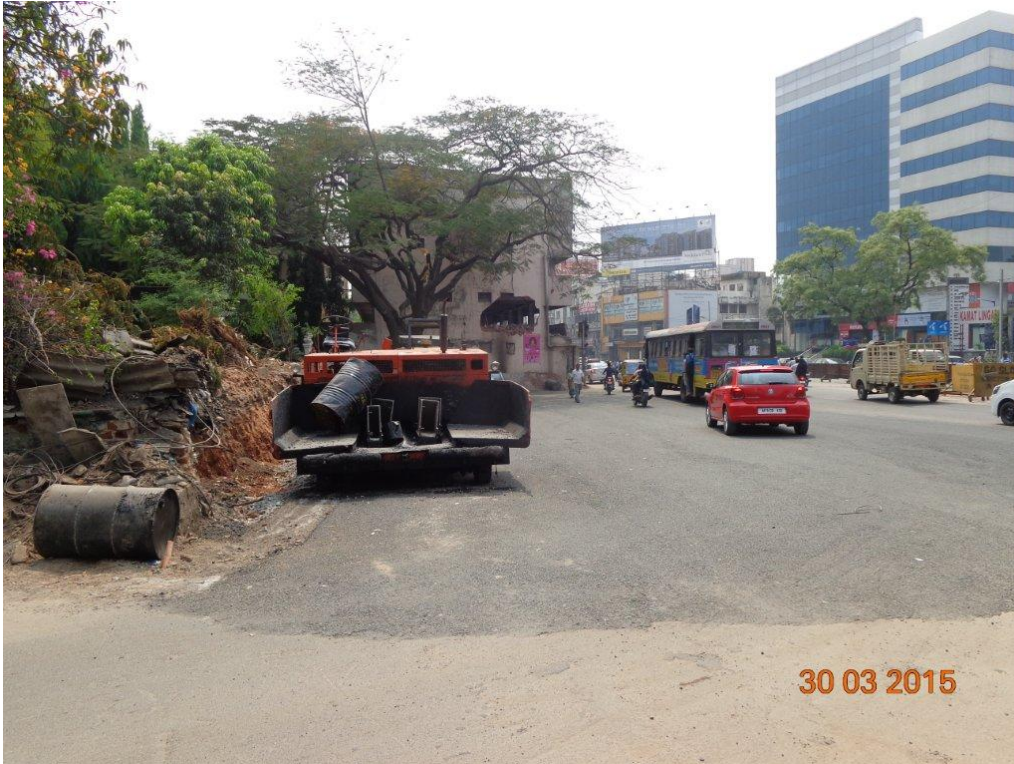
Formation of wide road in front of Allauddin building in Begumpet road
